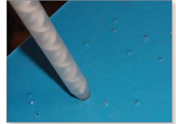
Figure 6: For short pot life urethanes, the material is simultaneously mixed and injected.
